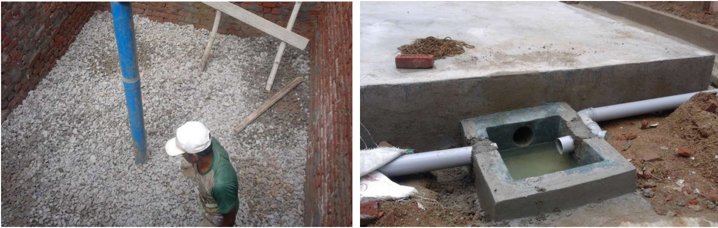
One of the water harvesting systems
