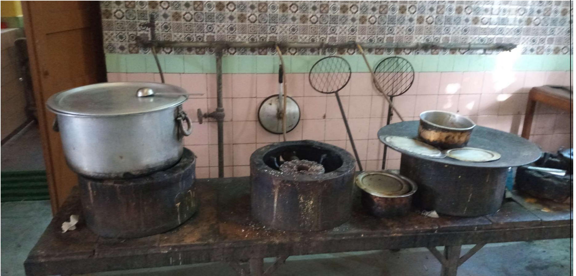
Biogas used kitchen purpose
